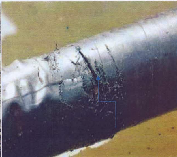
HACKSAW CUT ON THE FACILITY AT 12 O'CLOCK POSITION (AFTER EXCAVATION)
